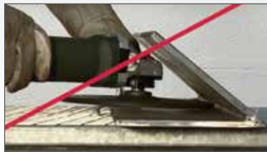
This solution violates safety standards
